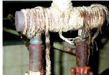
Amianto in cordonature
